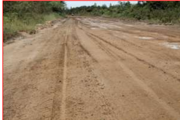
Hauling road condition
