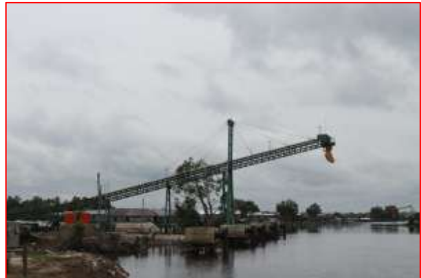
Conveyor belt at jetty
